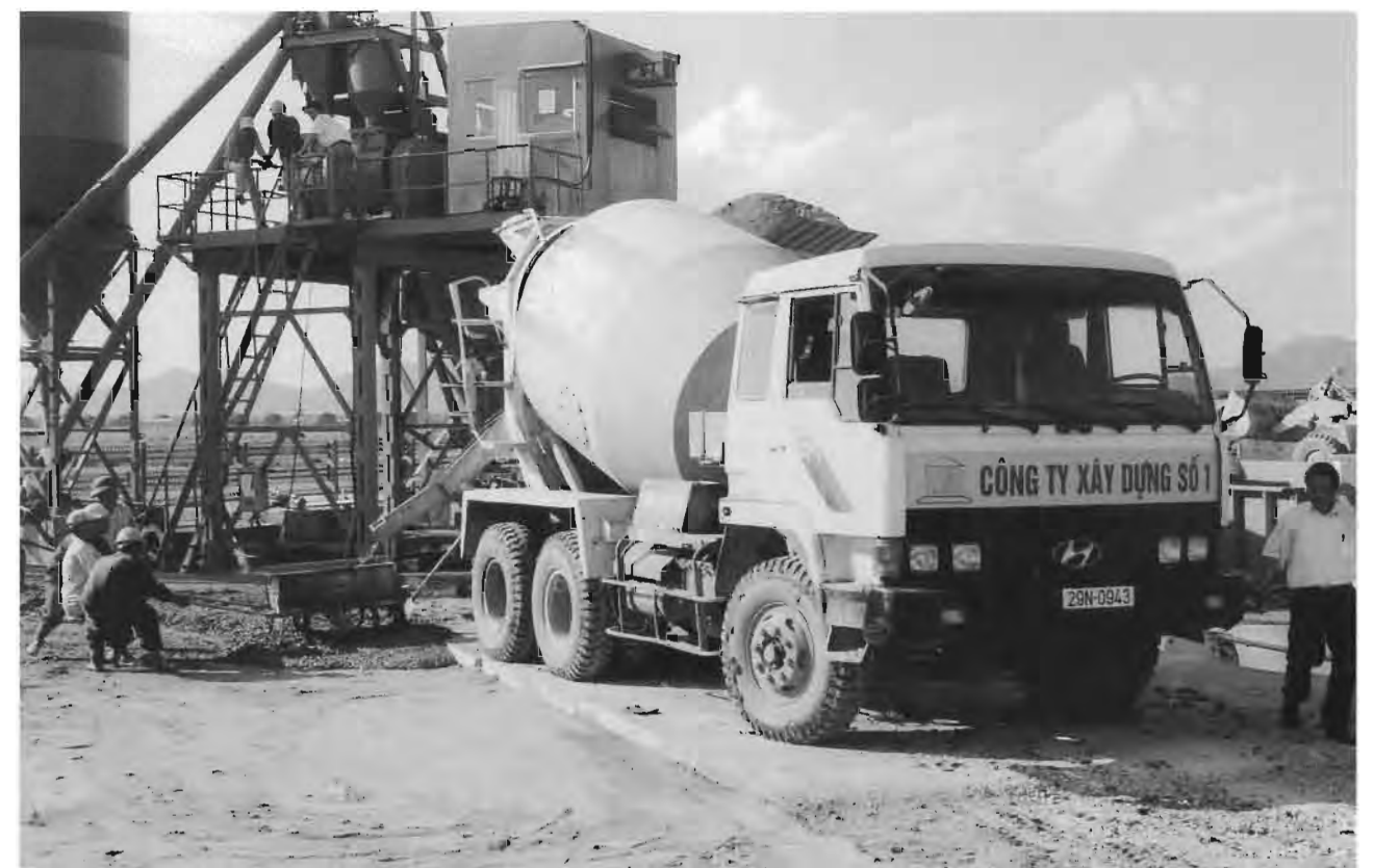
Trạm trộn bê tông - Concrete mixing station
