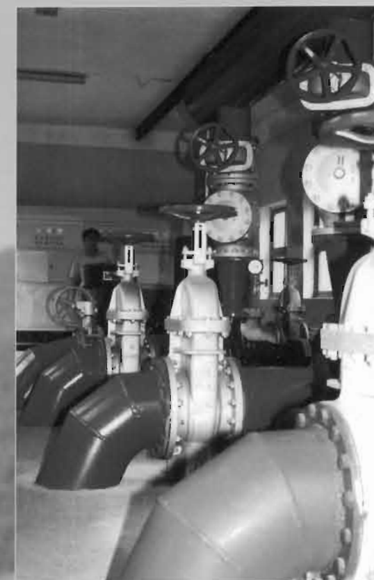
Trạm bơm nước sạch. Pumping Station.
