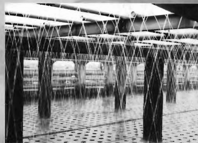
Xử lý nước. Water treatment.
