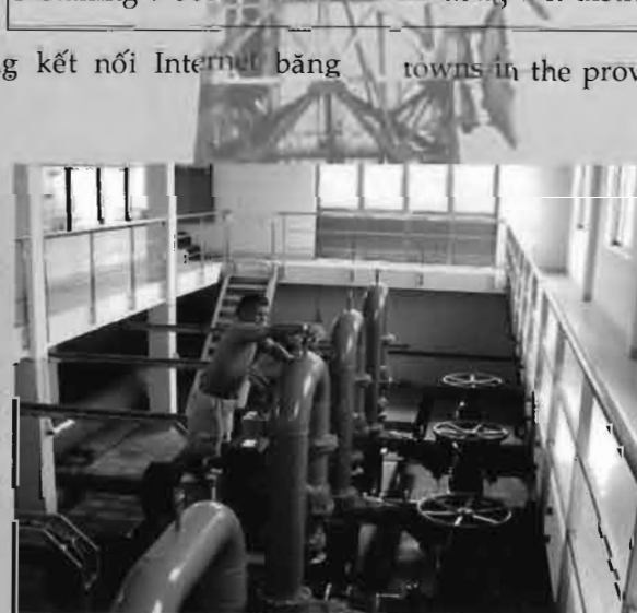
Operating the Son Tay Water Plant
