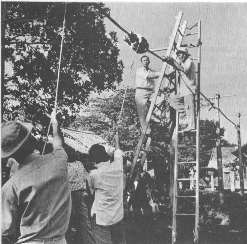
A line construction class learns to lash telephone cables together with a "spinner".
