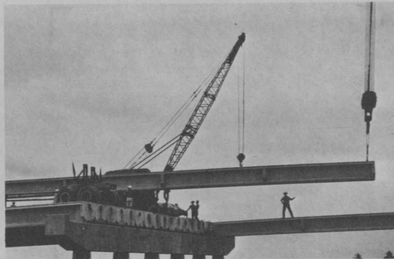
Bridges are under construction on the Bien Hoa highway as part of the rehabilitation and modernization of the transport system.
