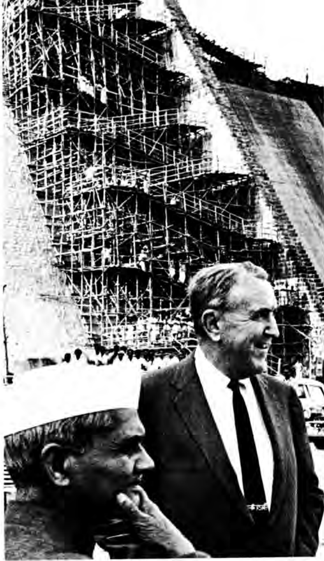
Sharavathi hydroelectric project is inspected by Ambassador Chester Bowles and India's late Prime Minister Lal Bahadur Shastri. The project, largest in South Asia, has received $102 million in U.S. aid and will ultimately produce 1.2 million kilowatts.
