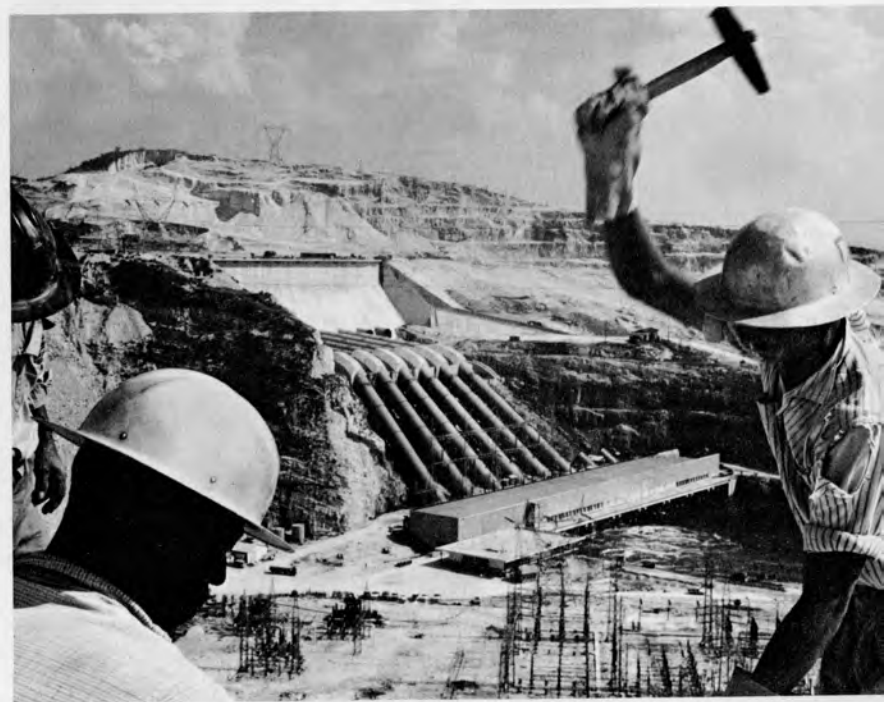
An important Alliance for Progress development is the Furnas Hydroelectric Power Project in Brazil.
