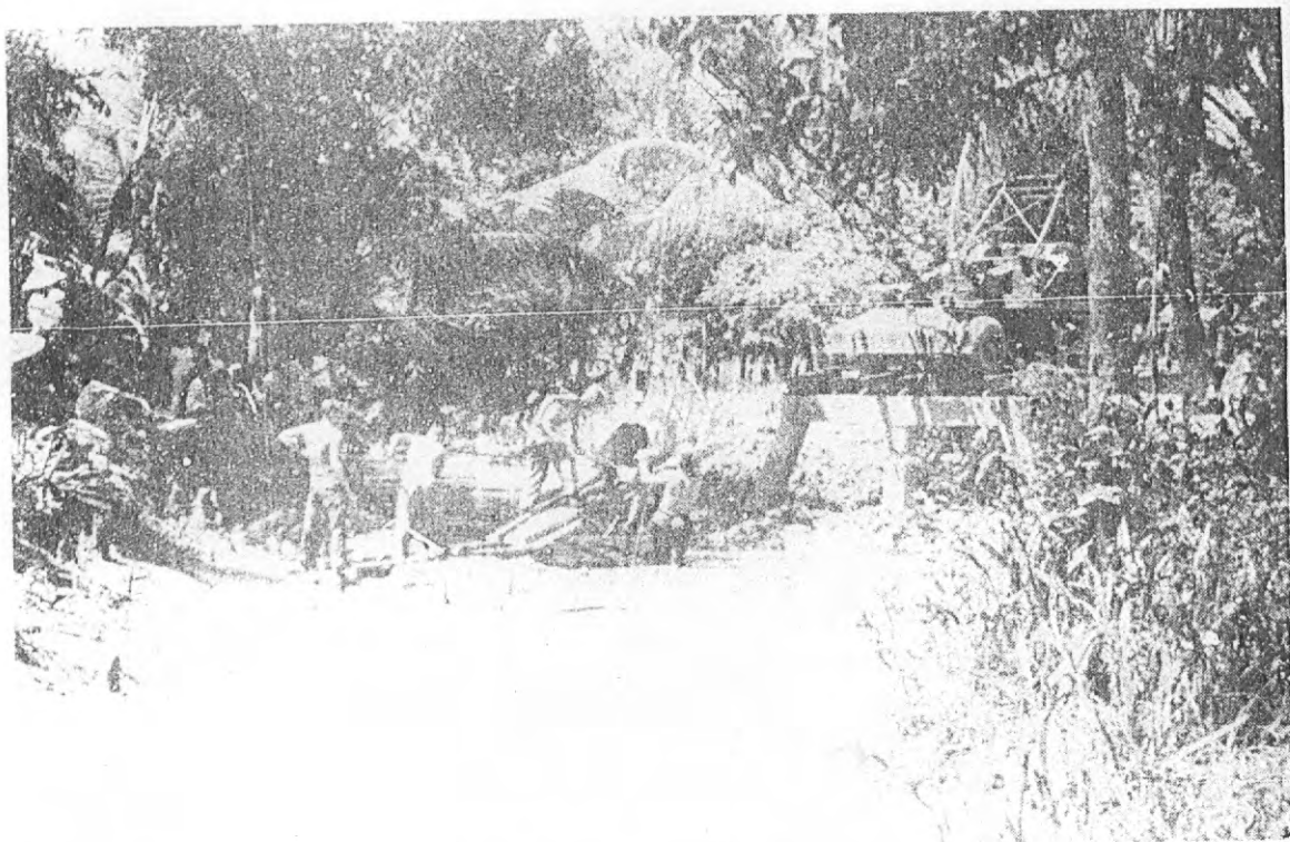
Members of Seabee Team 1009 prepare a concrete foundation for a foot bridge in a hamlet west of Vinh Long.
