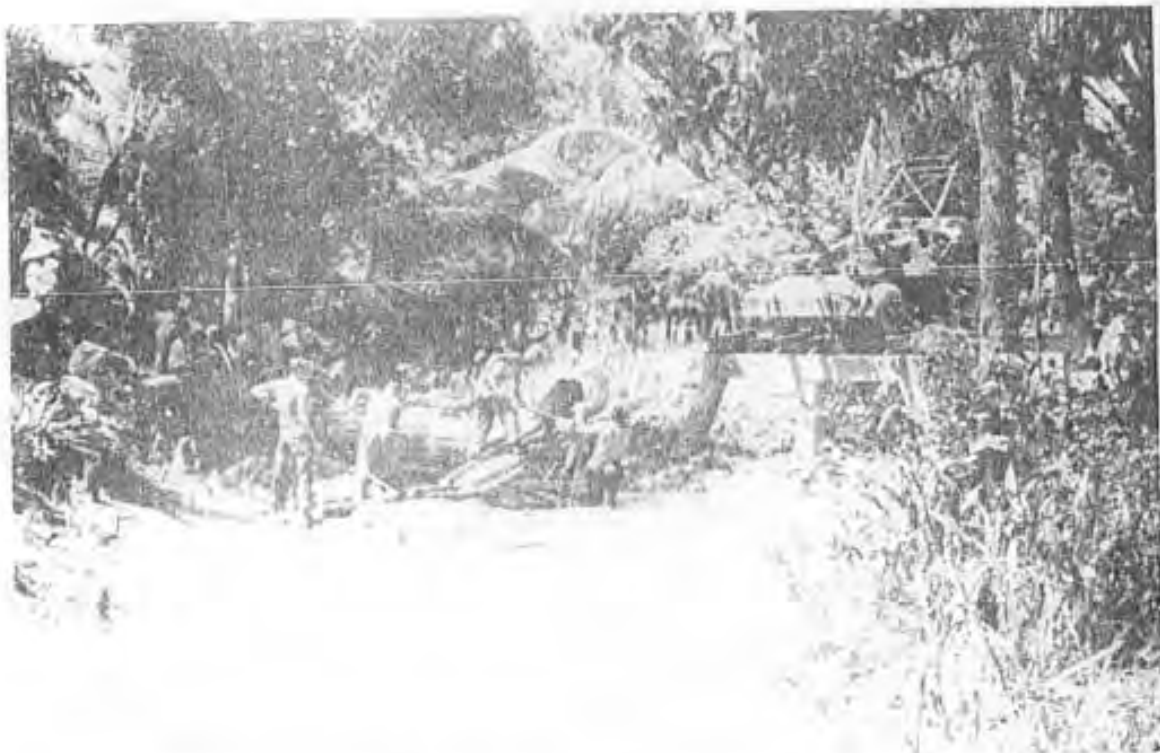
Members of Sumbawa Team 1009 prepare a concrete foundation for a foot bridge in a barlet west of Vinh Long.
