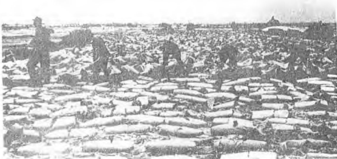
Seabees spread cement used to produce a soil base for the new airstrip at Long Ha.
