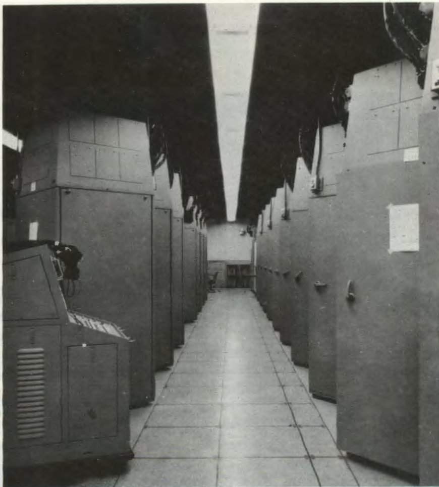
Figure 19. Data processing subsystem digital racks at the MSR.
