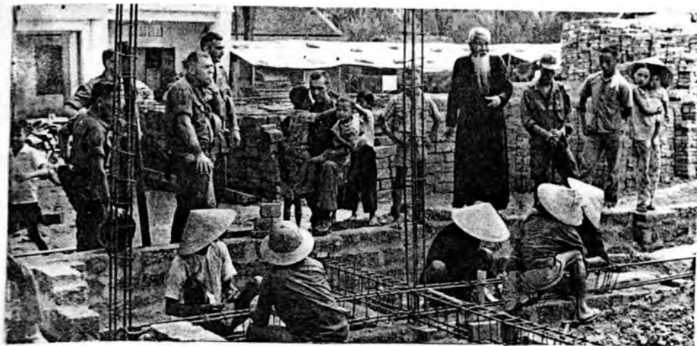
Father Bui Duc and members of the 1st Brigade check progress on the construction of Bong Son Refugee Center.
