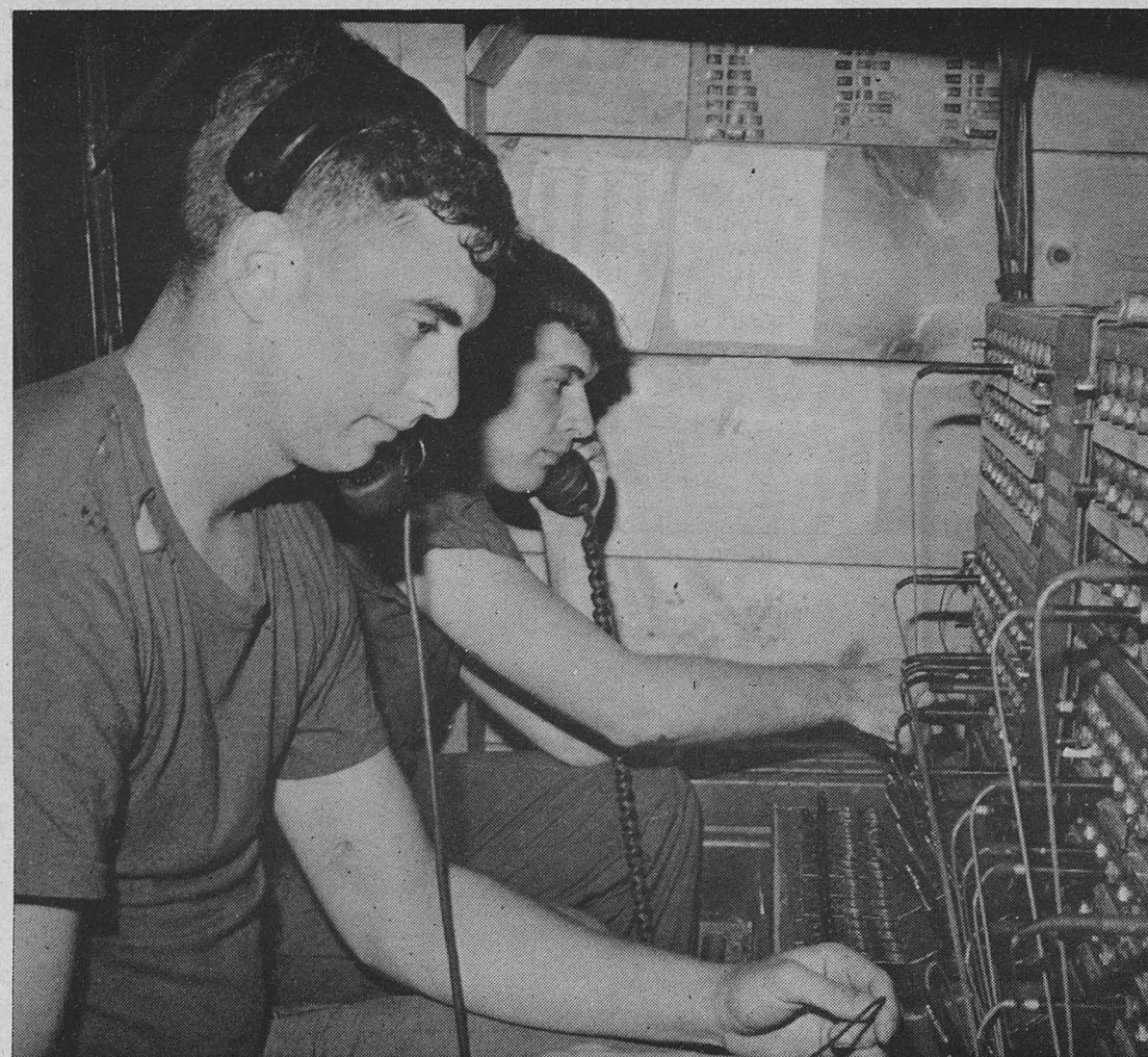
Switchboard operators at the Skyking switch prepare to break down their calls and resume the job of answering as 'Skyking, Sir.'
