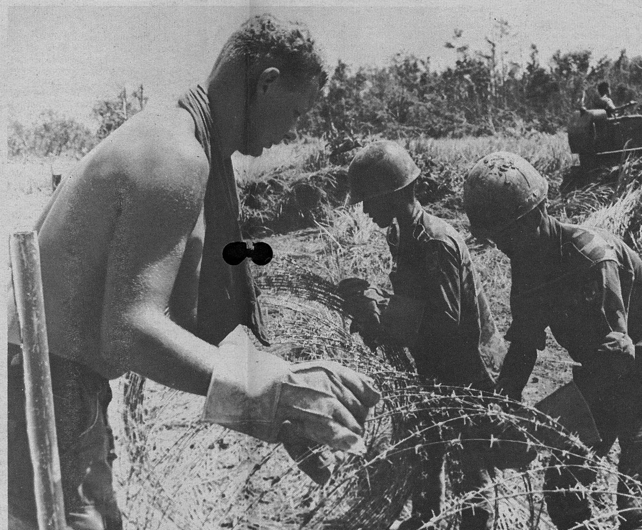
PFC Wayne Boss leads an ARVN work detail in setting up perimeter wire at FSB Jackie. Fifty combat engineers from Alpha Company, 8th Engineers helped the ARVN paratroopers establish their first fire support base.
