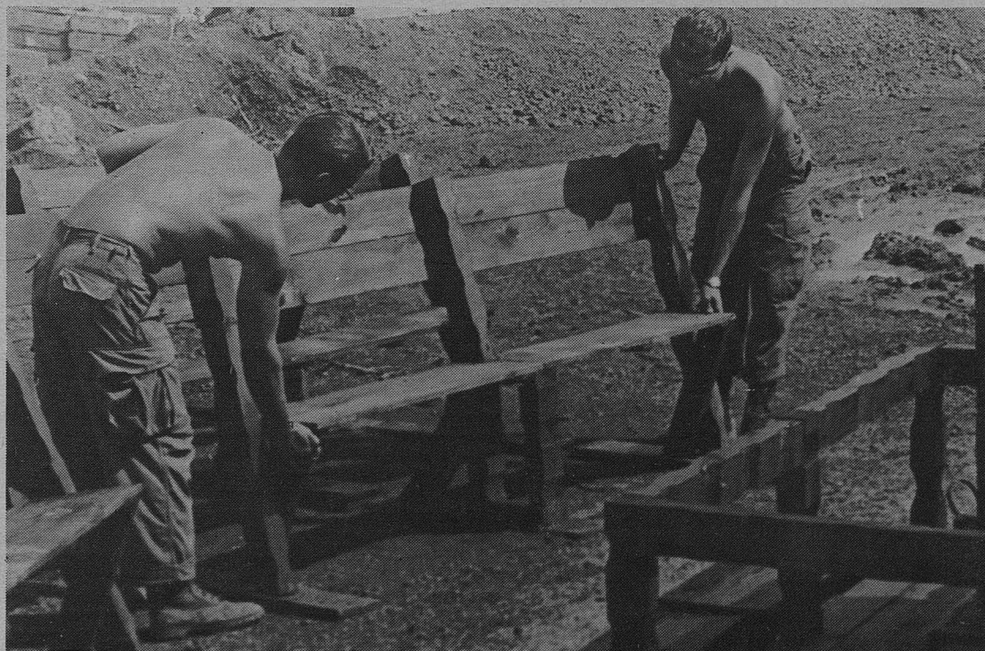
(U.S. Army Photo by PFC James McCabe) Specialists Four John Pitt (left) and Gary Bradley set pews in place during the construction of an outdoor chapel by members of Battery A, 1st Battalion, 21st Artillery. The 1st Air Cavalrymen are located at Fire Support Base Mary.
