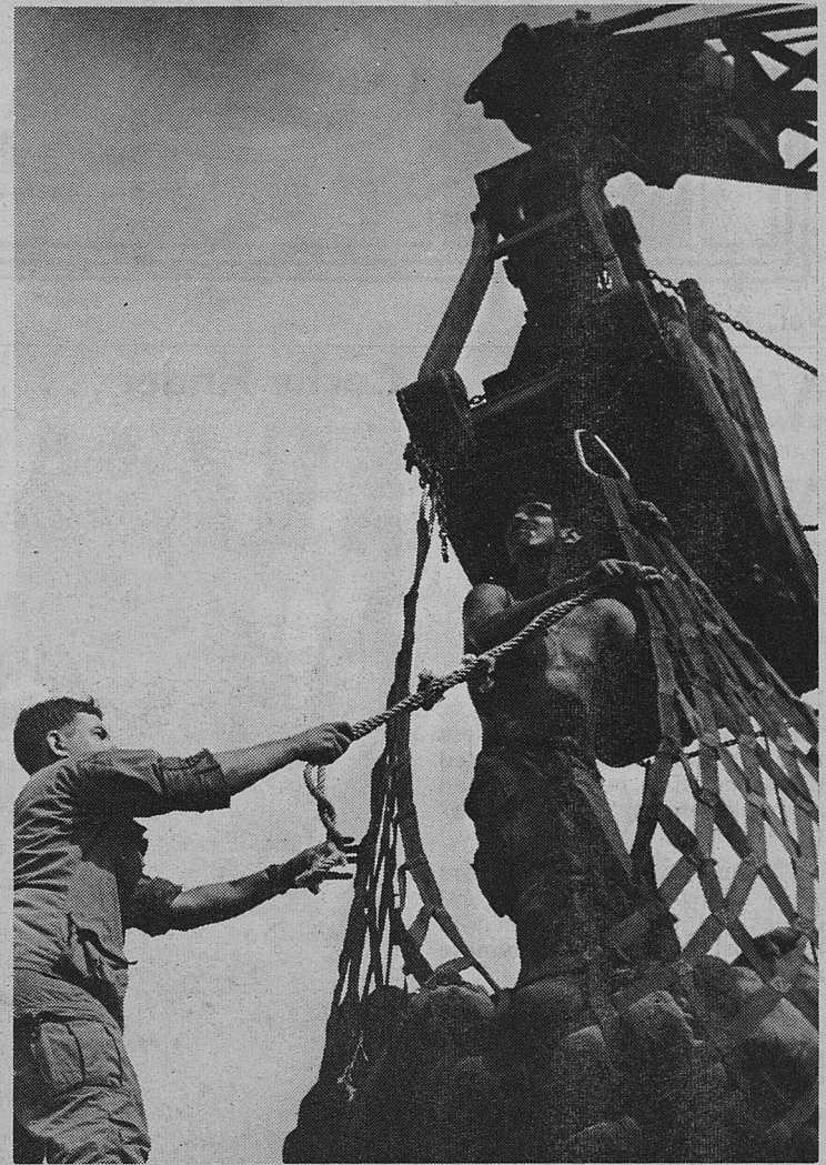
(U.S. Army Photo by PFC James McCabe) Second Lieutenant Robert Krause (left) and Sergeant Thomas Gutierrez, both of Company B, 8th Engineer Battalion, guide a load of sandbags to the roof of the TOC (Tactical Operations Center) at Fire Support Base Buttons, home of the 1st Air Cav's 2nd Brigade.
