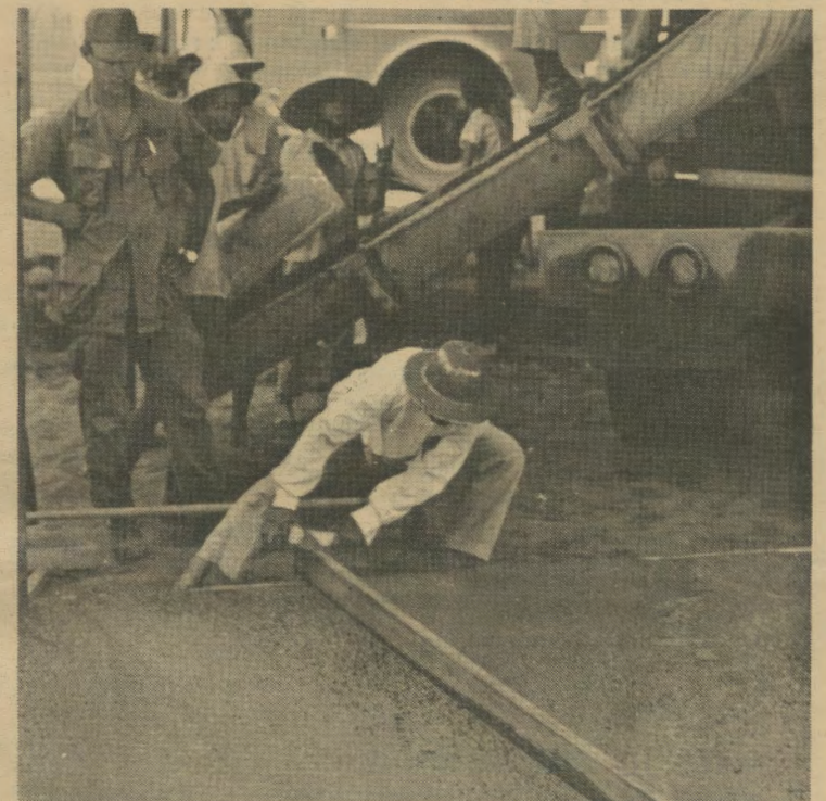
A Vietnamese worker levels a section of concrete as work on the floor of a new marketplace for the village of Hoa Vang progresses. Airmen from the 366th Civil Engineering Squadron assisted the Vietnamese in the project.
