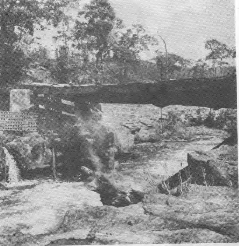
Dai Don bridge in Phu Son village blown up by the VC. After this act of sabotage, the bridge was unusable and the villagers had difficulties taking their produce to market.
